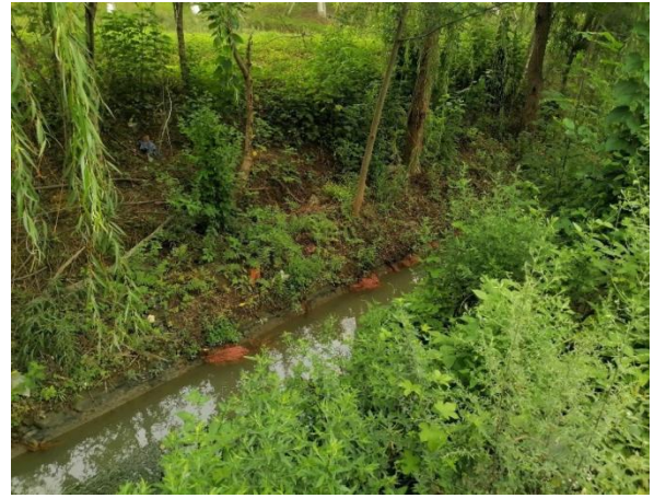
渠道破损，渗漏
